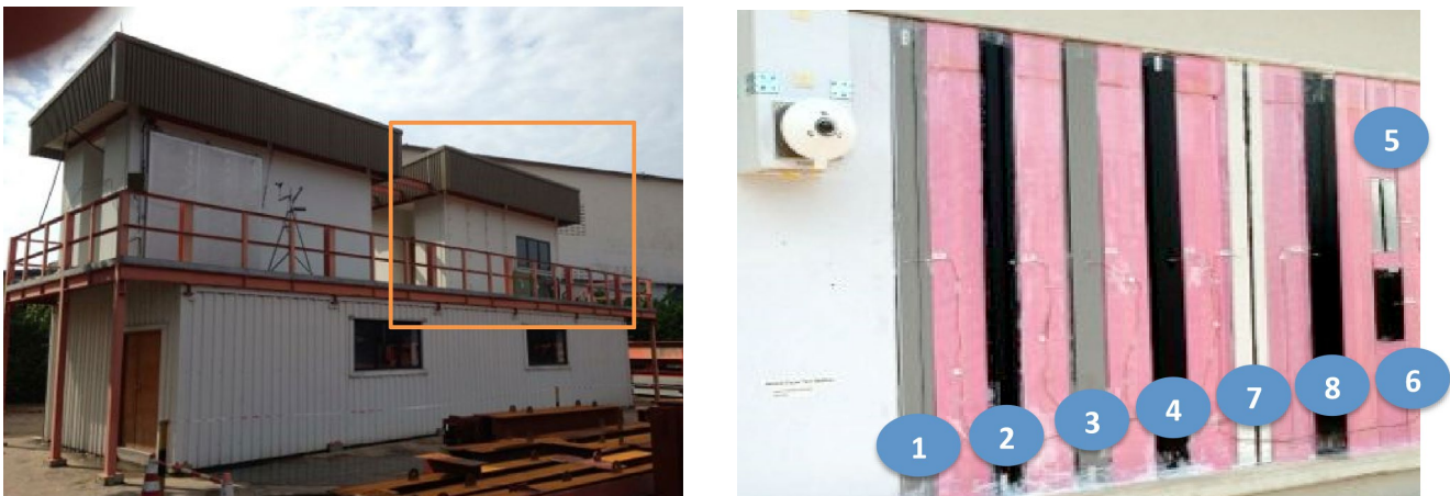
Figure 2: The conditioned test room (left) and a close-up of the framing members in the wall of the test hut (right).
